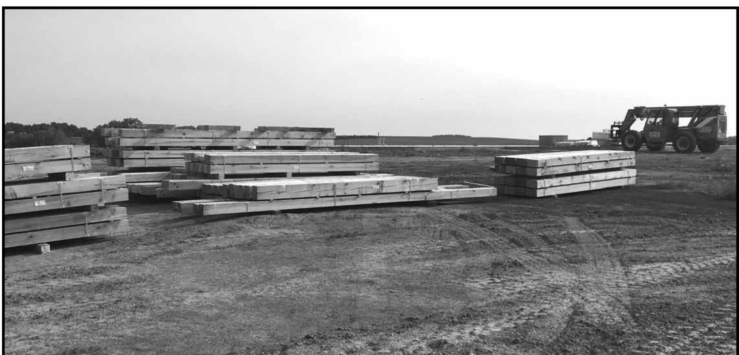
The barn kit for the 15,000 square-foot facility was delivered Wednesday morning to the site where crews began to unload and organize the timbers. (Contributed images)
